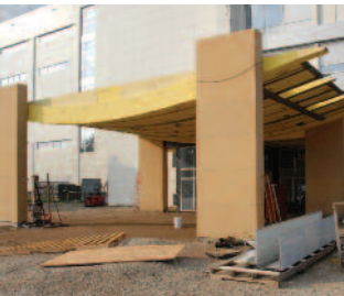
The canopy over the Emergency Department entrance mimics the graceful arc that's the signature design of the hospital's main entrance.
